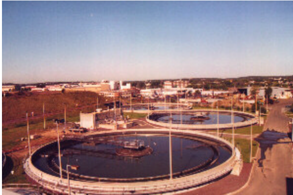
Secondary clarifiers in a wastewater treatment plant
