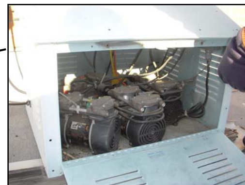
IMPROVE Pumping Unit
